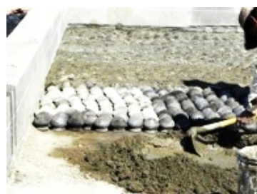
Figure 1. Local potters laying 20,000 clay pots to create thermal buffer on the roof. (Photo Credit: Artha Studio)
